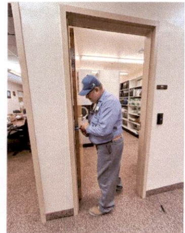
Alignment of a door at the City Hall.
